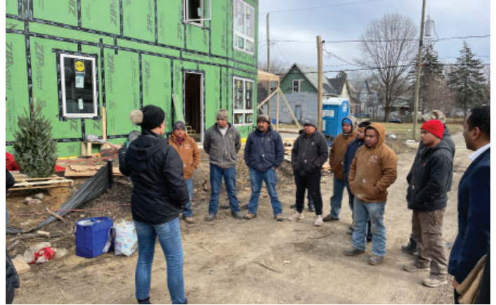
Students and Framing Crew Joined to Celebrate The Project With A “Topping Out” Celebration (2022)
